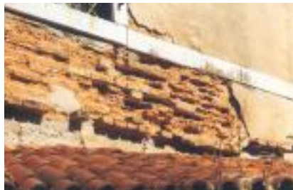
Venice: salt damage to brickwork and plaster.
